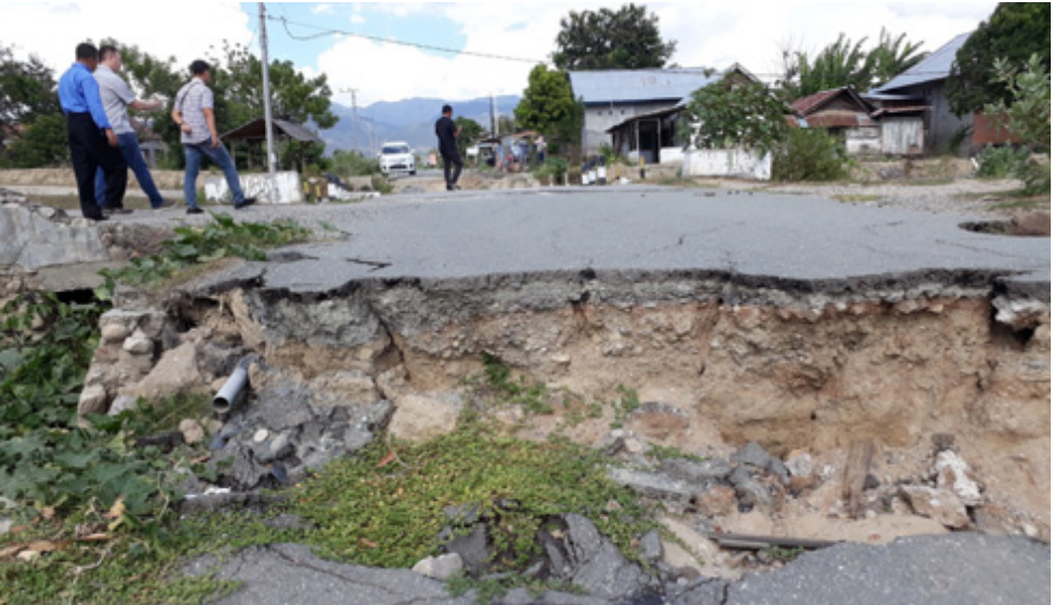
Connecting roads to and from affected areas destroyed by the earthquake. Image Source: Angelo Paolo L. Trias.
