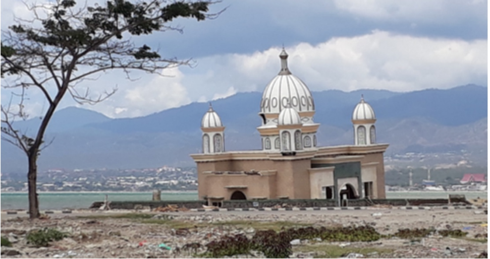
Mosque and other structures along the coast of Palu damaged by the tsunami. Image Source: Angelo Paolo L. Trias.
